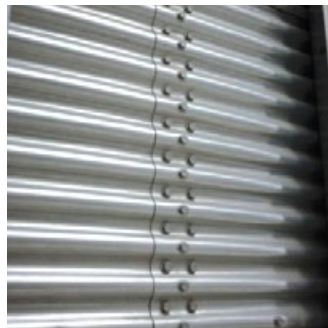
ENG. Detailed view of the junction between sheets FRA. Détail jonction viroles
