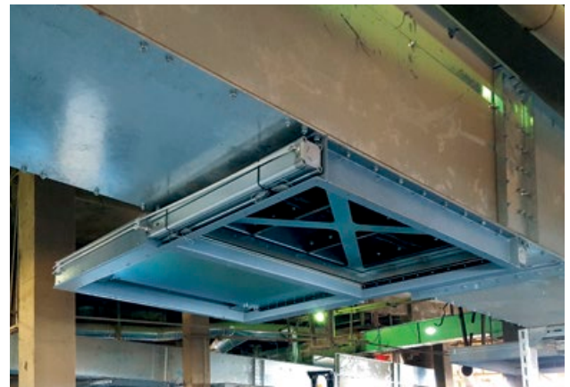
Detailed view of unloading shutter
